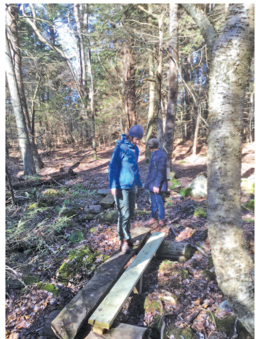
Trail Steward, Diane Jakobsen, and volunteers repairing the bog bridges on Hurlbut Field Trail to Winchester Lake
